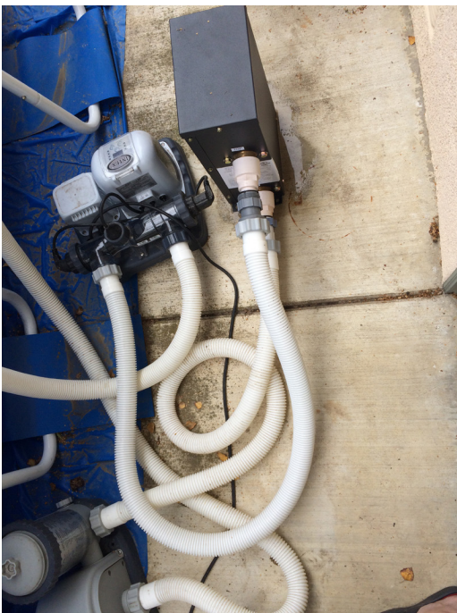
Saltwater System with Heater
